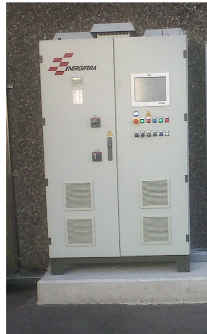
QC - quadro controllo
