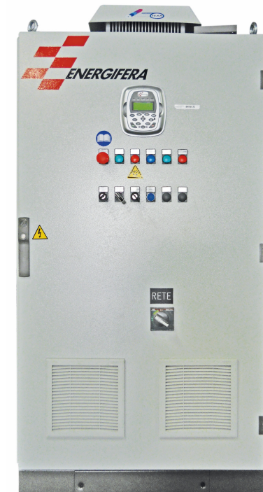
QC – quadro controllo
